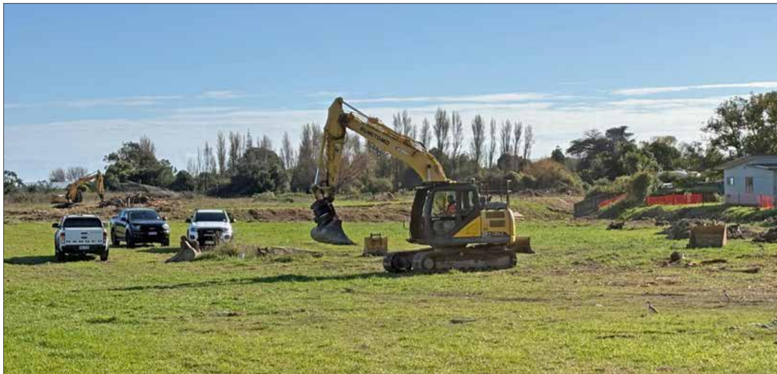
Heavy machinery seen on May 11 signals the beginning of work at Moy Estate.
