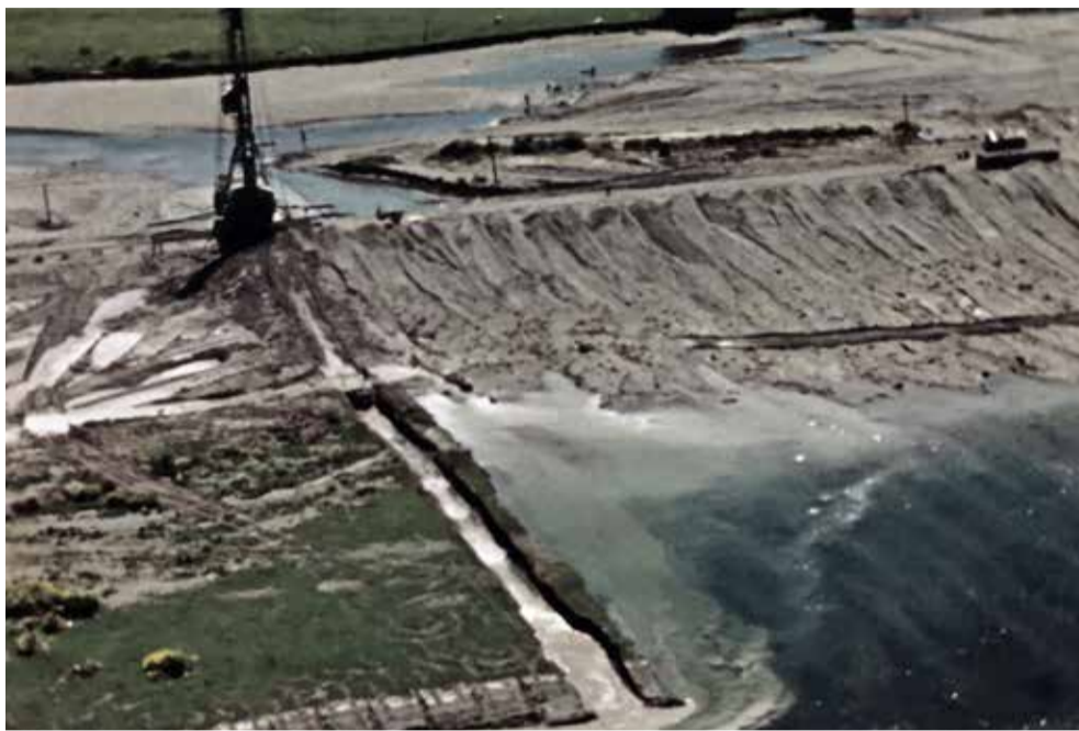
The huge Tower Dredge at work on the Ōtaki River in 1946. The image is from a video held by Ngā Taonga Sound & Vision. To view, search “Ōtaki Dragline” at ngataonga.org.nz
